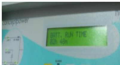
Gbr. 6 Dokumentasi Backup time
